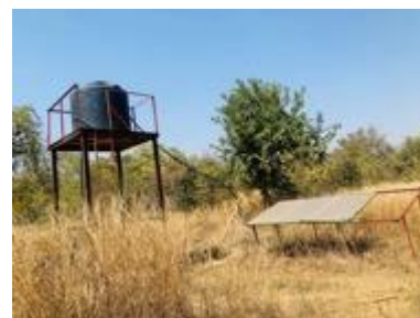
1000-liter water tank and 3 school panels with metal brackets
